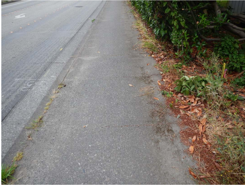
Photo 3. View north on Yew Street of northwest property corner, sidewalk, curb, and gutter.
